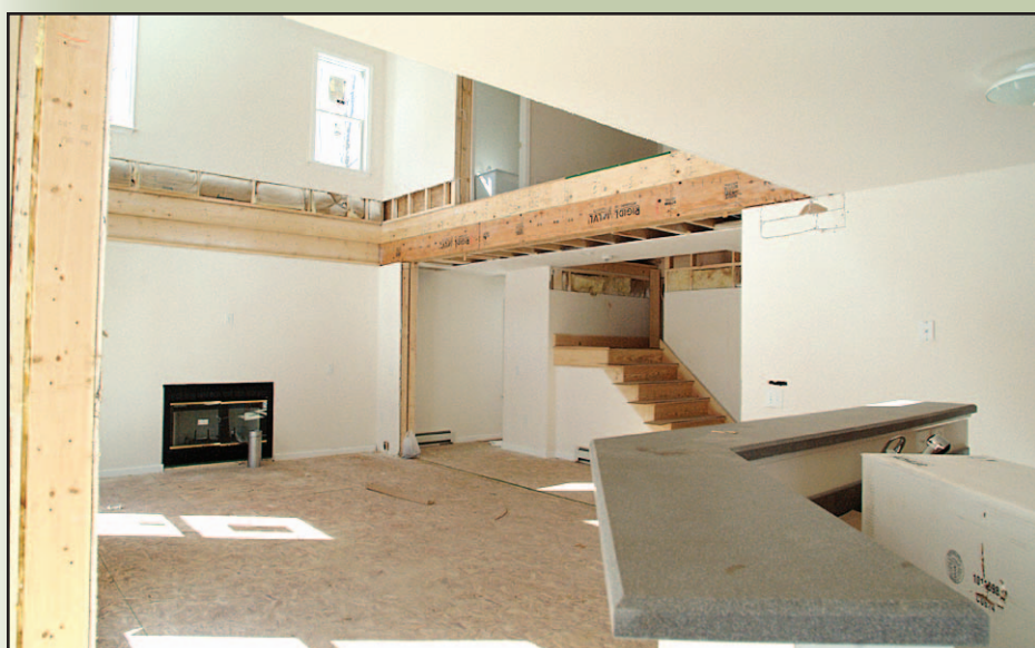
Inside divisions between first and second floor pre-fabricated sections can be seen where sheet rock has not yet been attached. The kitchen countertops are crowned with Dupont Corian.
